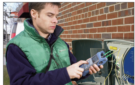
■ The PPM-352B-EG-ER used at the ONT.
